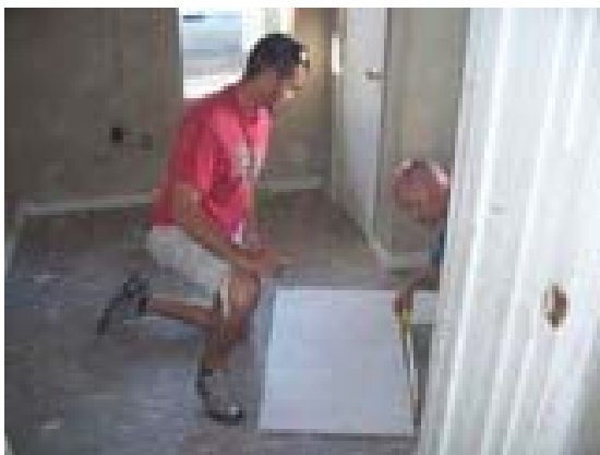
Murray State volunteer Alex Mulvaney (left) and CrossRoads team leader Jairus Durnett work on sheetrock for Alexandria's room.
