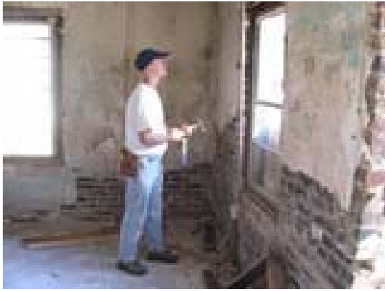
CrossRoads Church member Jairus Durnett examines the walls of the living room on the first work day in August 2010.
