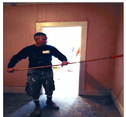
On the inside, new insulation & sheetrock were installed. Interior walls were finished and painted.
